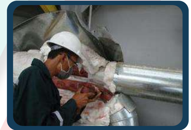
Preliminary Operation & Maintenance Assessment Dual Fuel Power Plant 2 x 63 MW in Berau, East Kalimantan
