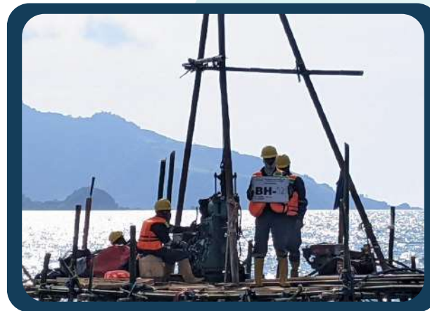
Soil Investigation, Topography & Bathymetry Survey for Jetty Facility of Coal Fired Power Plant in East Nusa Tenggara, Indonesia
