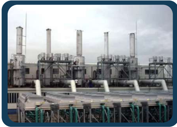
North Halmahera, Diesel Engine Power Audit
