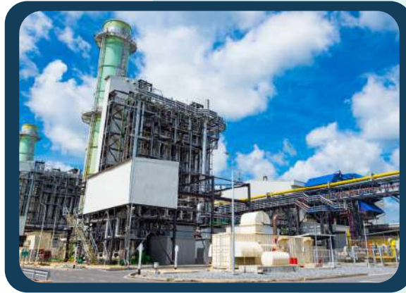
Remaining Life Assessment Boiler System of Sekayan Coal Fired Steam Power Plant 1 x 7,5 MW - North Kalimantan, Indonesia
