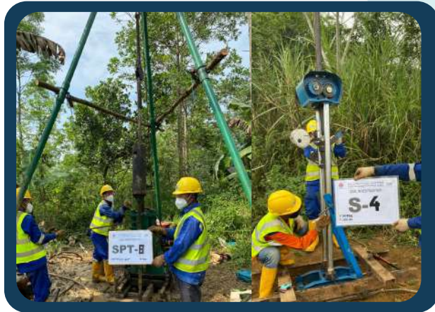
Soil Investigation for 32.5 MW Ground Mounted Solar PV Plant West Java, Indonesia
